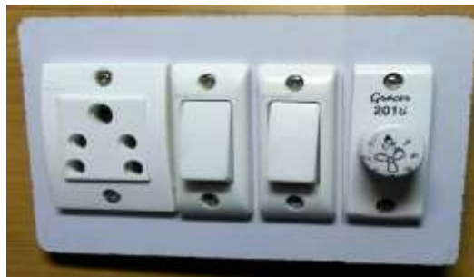
Figure: Switch Board
